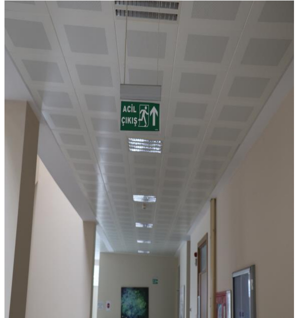
Emergency exit signs
