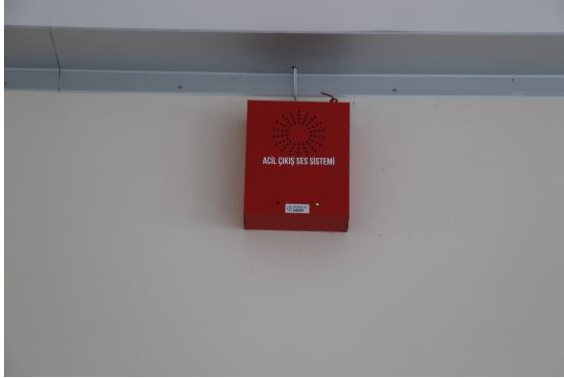
Emergency exit sound system
