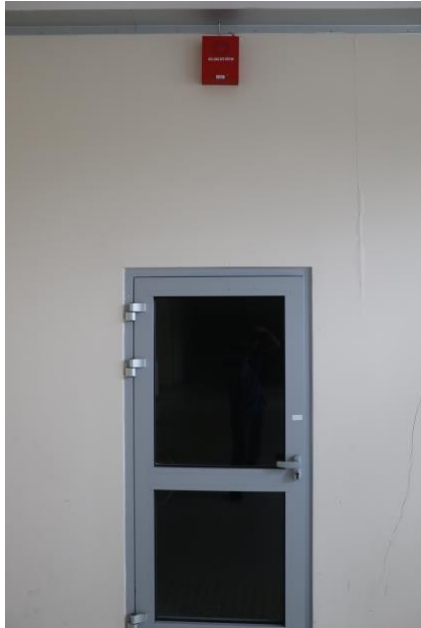
Emergency exit sound system and emergency exit door
