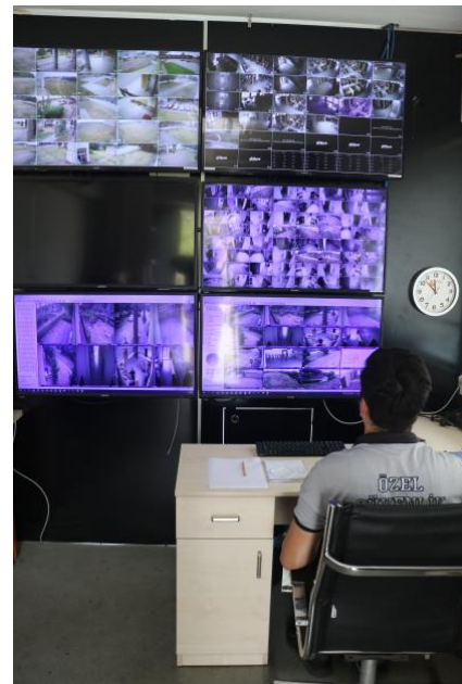
Security surveillance system
